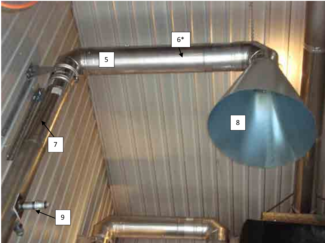
Picture 2 : Hood and mixing baffle
